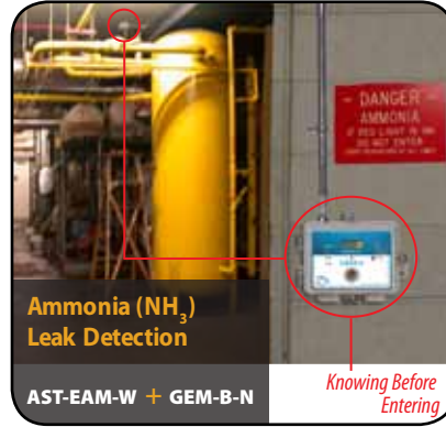
Arenas - Ammonia Compressors
