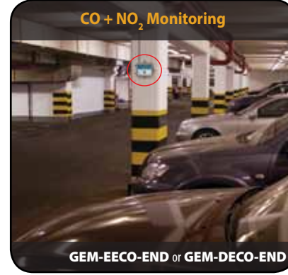
Parkades - Gas & Diesel Engine Exhaust
